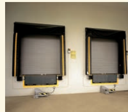
Rolling Service Doors
