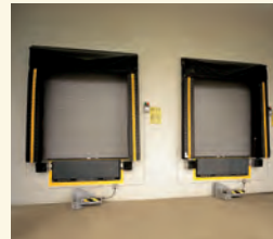
Rolling Service Doors
